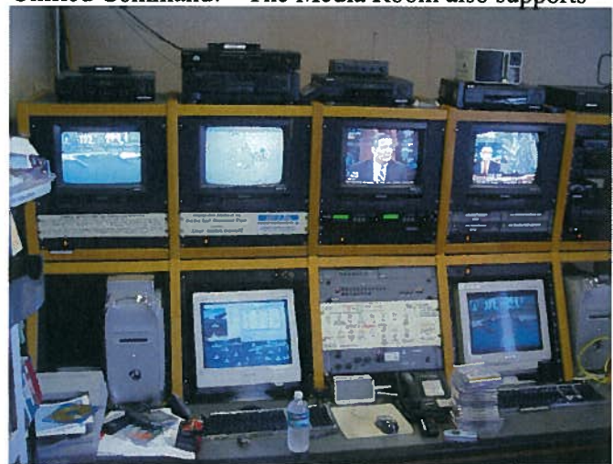
View of the Media Center control board.
